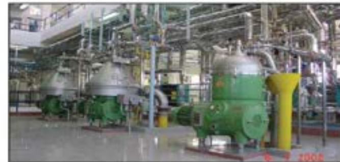
(i) A piping network in an industrial facility.
